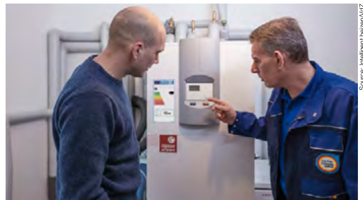
Source: Intelligent heizenVdZ
