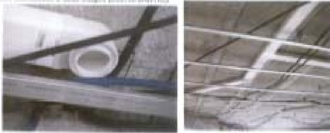
Figure 3-2: Example of ducts, Courtesy Atlantic- (CFP, 2006)
